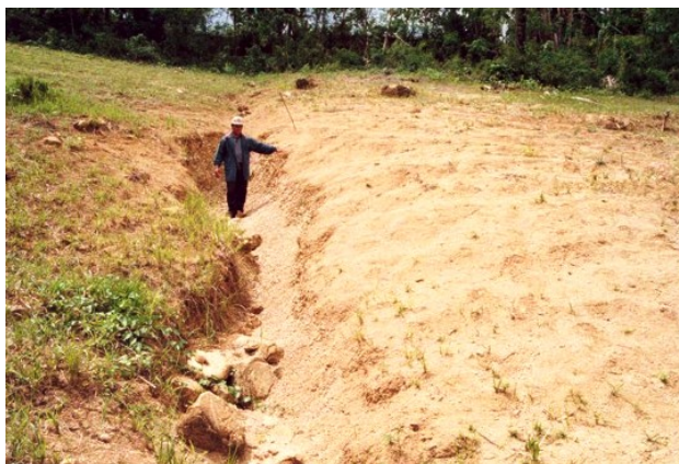
Photo 6.1. Soil erosion process on abandon sloping degraded areas form the study site
